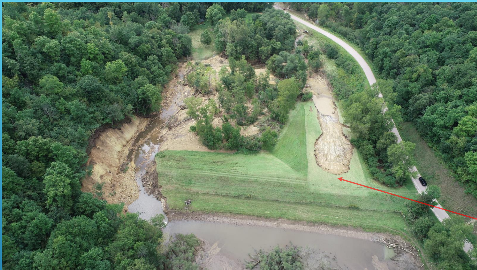
Left Abutment Breach - 25,000 cu.yds.
