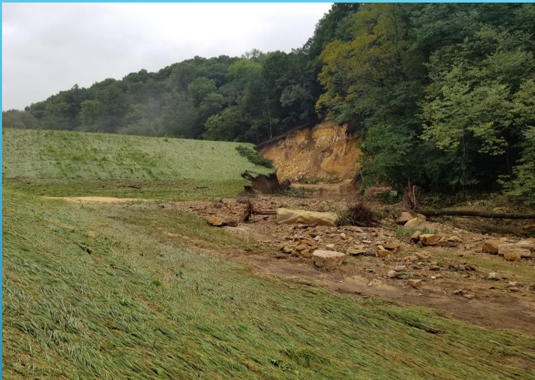
Left Abutment Breach -17,000 cu.yds.
