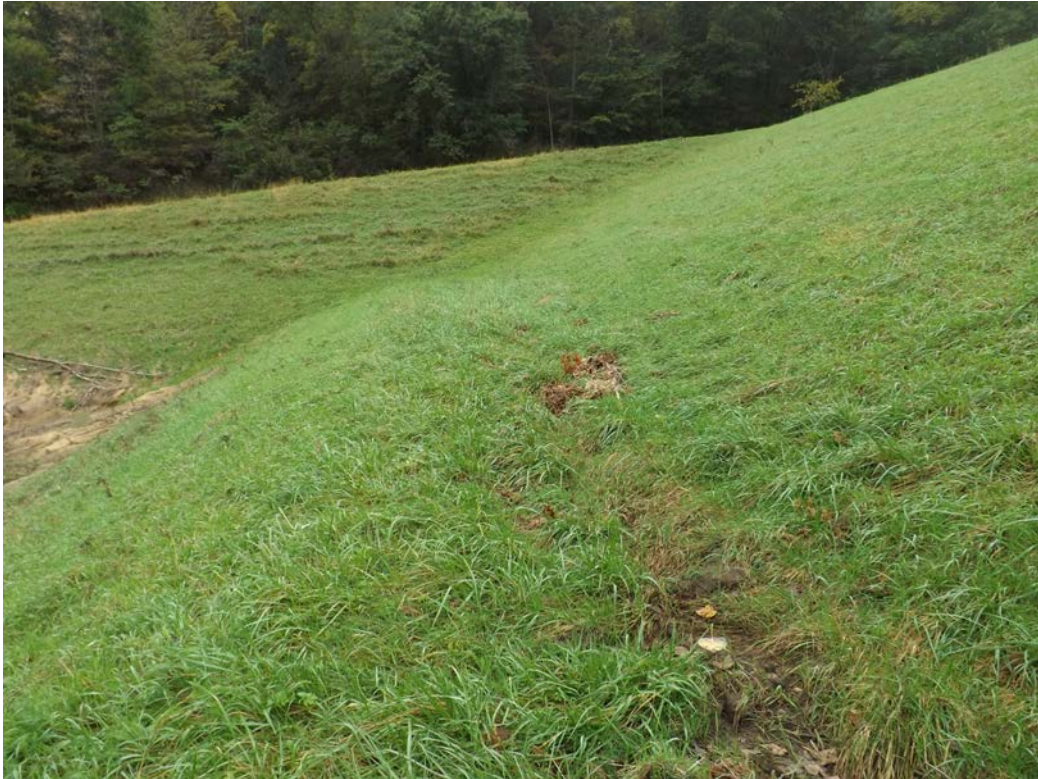
Photo 35 View of vegetation on downstream berm and embankment. (CC 21)
