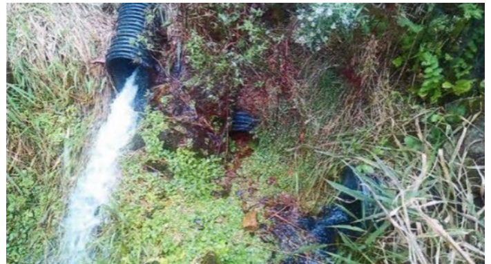
Seepage from Right Abutment Drains
