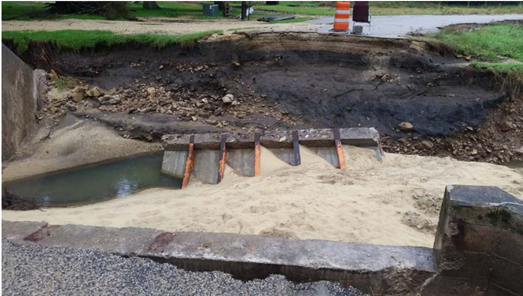
Photo 59 Remnants of county bridge downstream of house. (CC 23)
