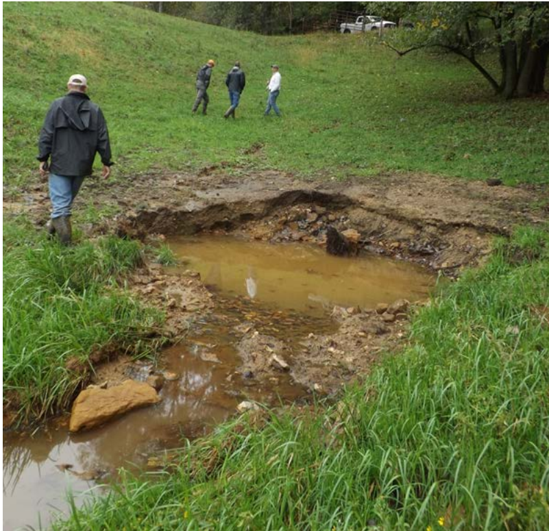
Photo 16 Scour hole at toe of left downstream groin. (WFK MLSNA)
