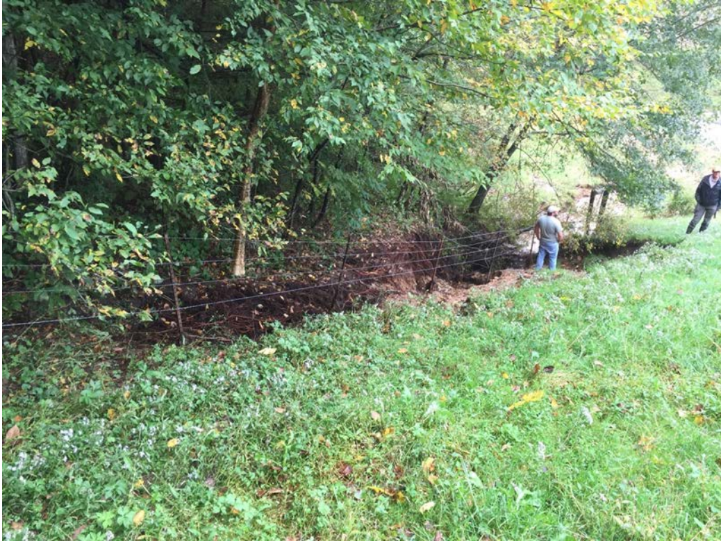
Photo 32 View of erosion in left groin from top of dam. (WFK 3)
