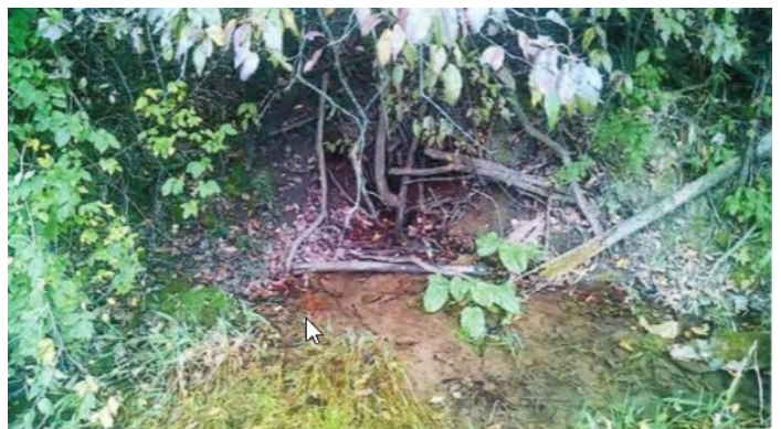
Seepage from Right Abutment Bedrock
