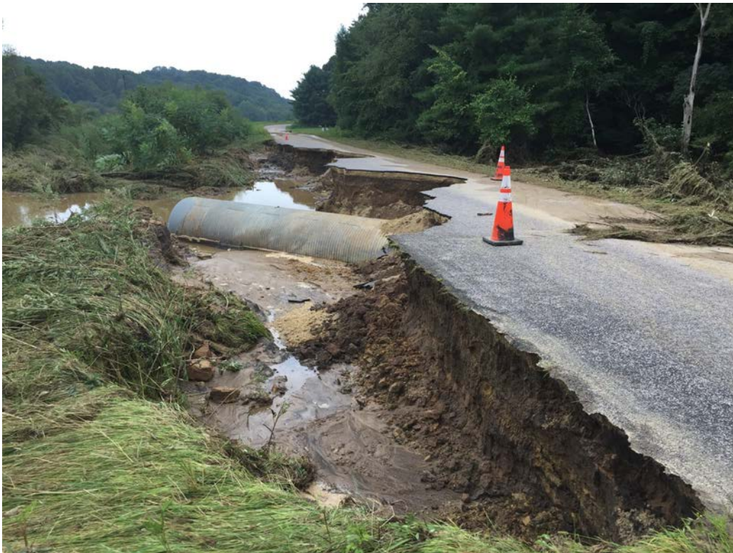
Photo 25 Damaged road in breach inundation area. (WFK MLSNA)
