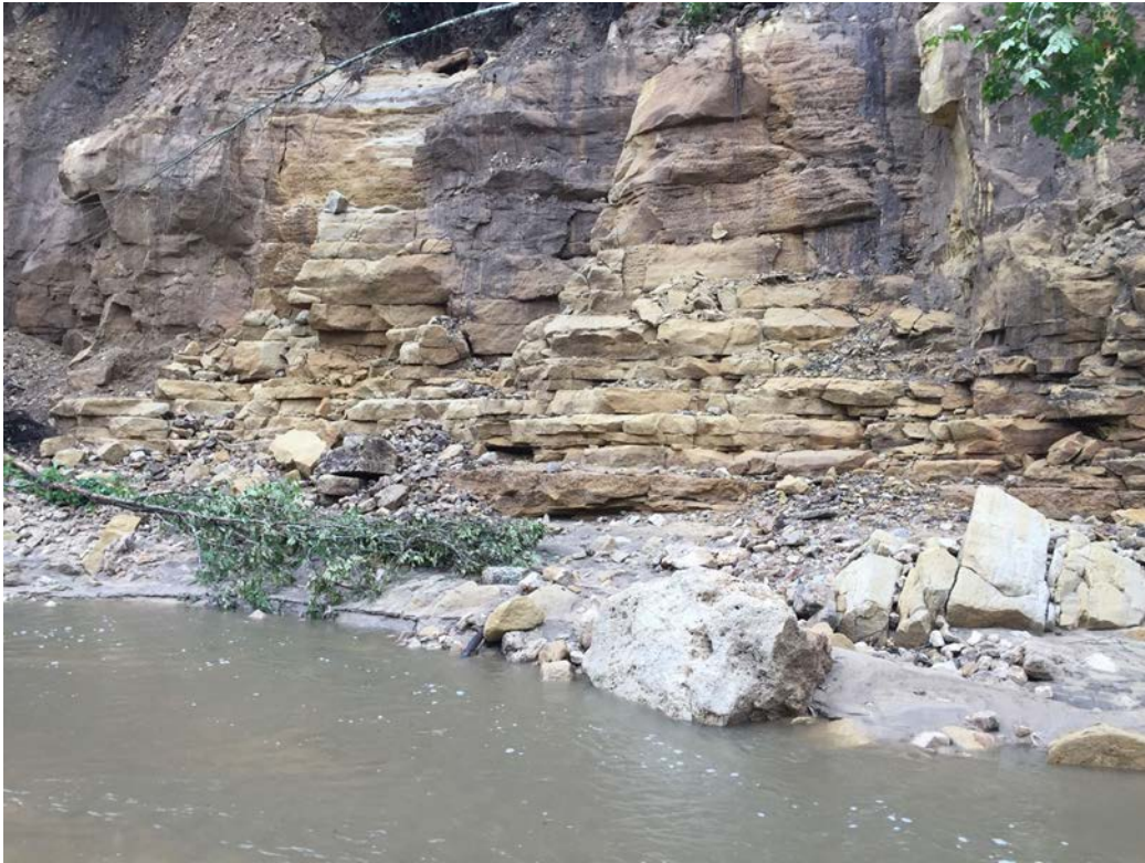
Photo 40 View of exposed bedrock in breach channel from near upstream toe of dam. (CC 21)
