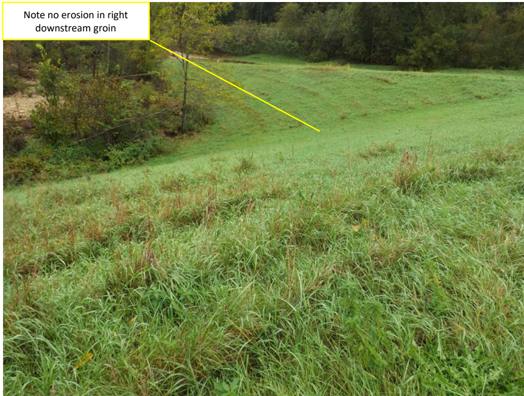
Photo 43 View of downstream embankment and auxiliary spillway dike vegetation from top of dam. (CC 29)
