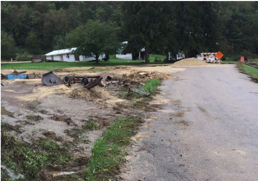
Photo 57 View of ranch house and bridge washout from county road. (CC 23)
