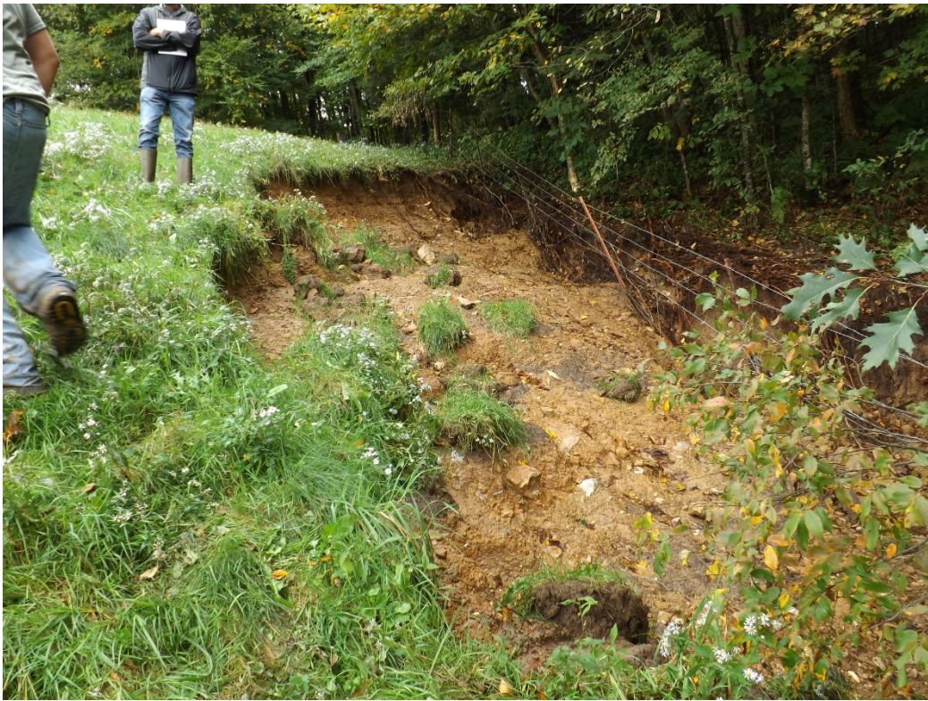
Photo 33 Erosion in left groin. (WFK 3)
