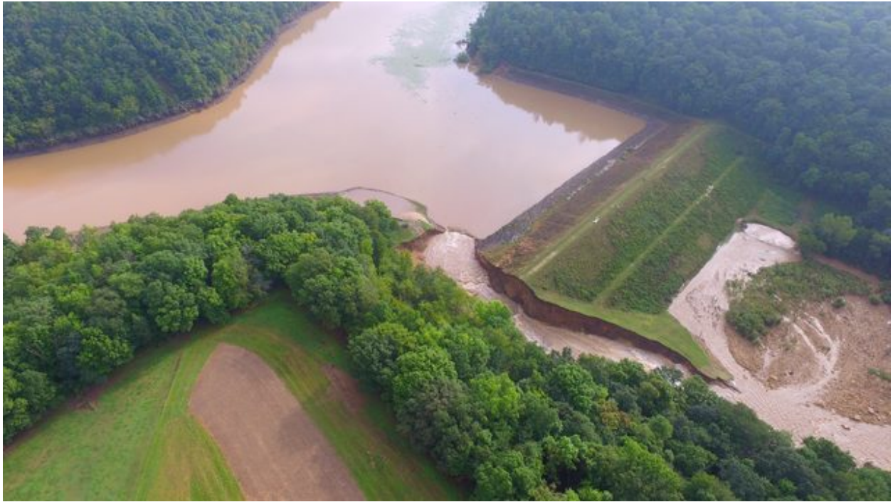
Photo A1 Aerial View of WFK 1 following breach on August 28, 2018
