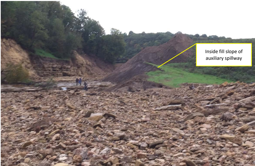
Photo 12 View of breach channel and left end of dam from downstream of dam. (WFK 1)
