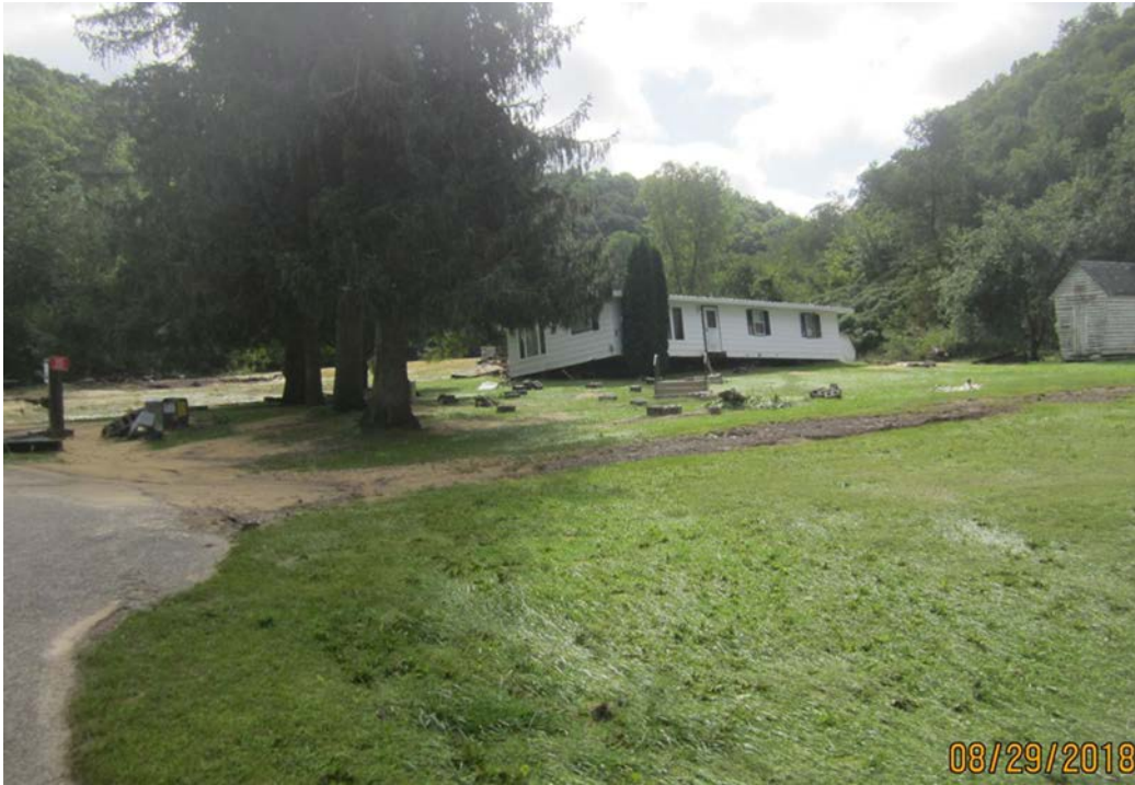
Photo 58 View from downstream county road of damaged house in breach inundation area. (CC 23)
