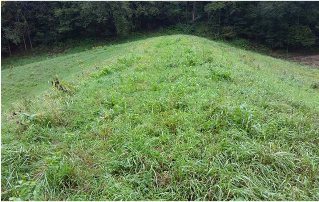
Photo 56 View of top of embankment from top left end of dam. (CC 23)
