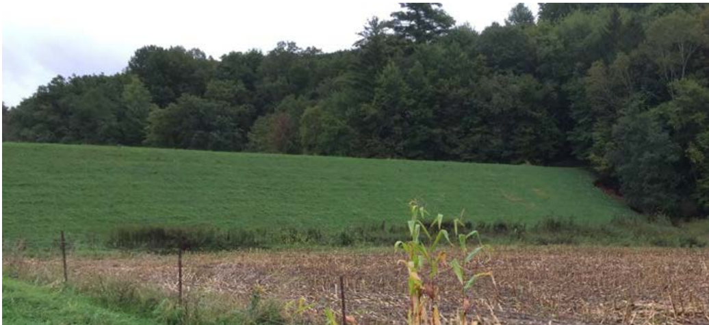
Photo 29 Downstream side of embankment. Vegetative cover did not fail during over-topping. (WFK 3)
